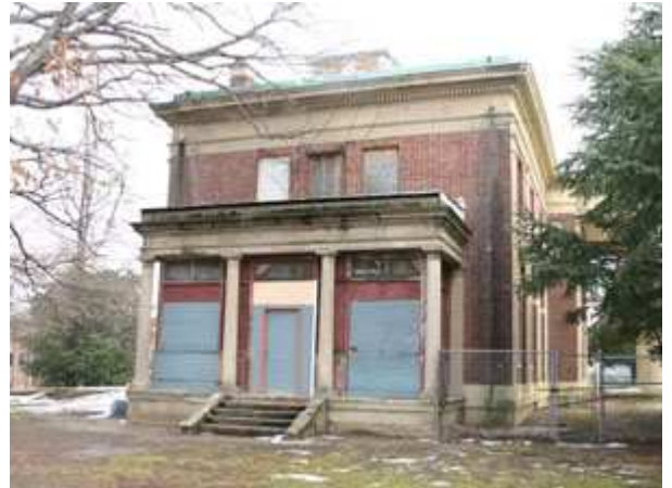
Ward Bucher The mansion was in a serious state of disrepair when the restoration program was initiated.
