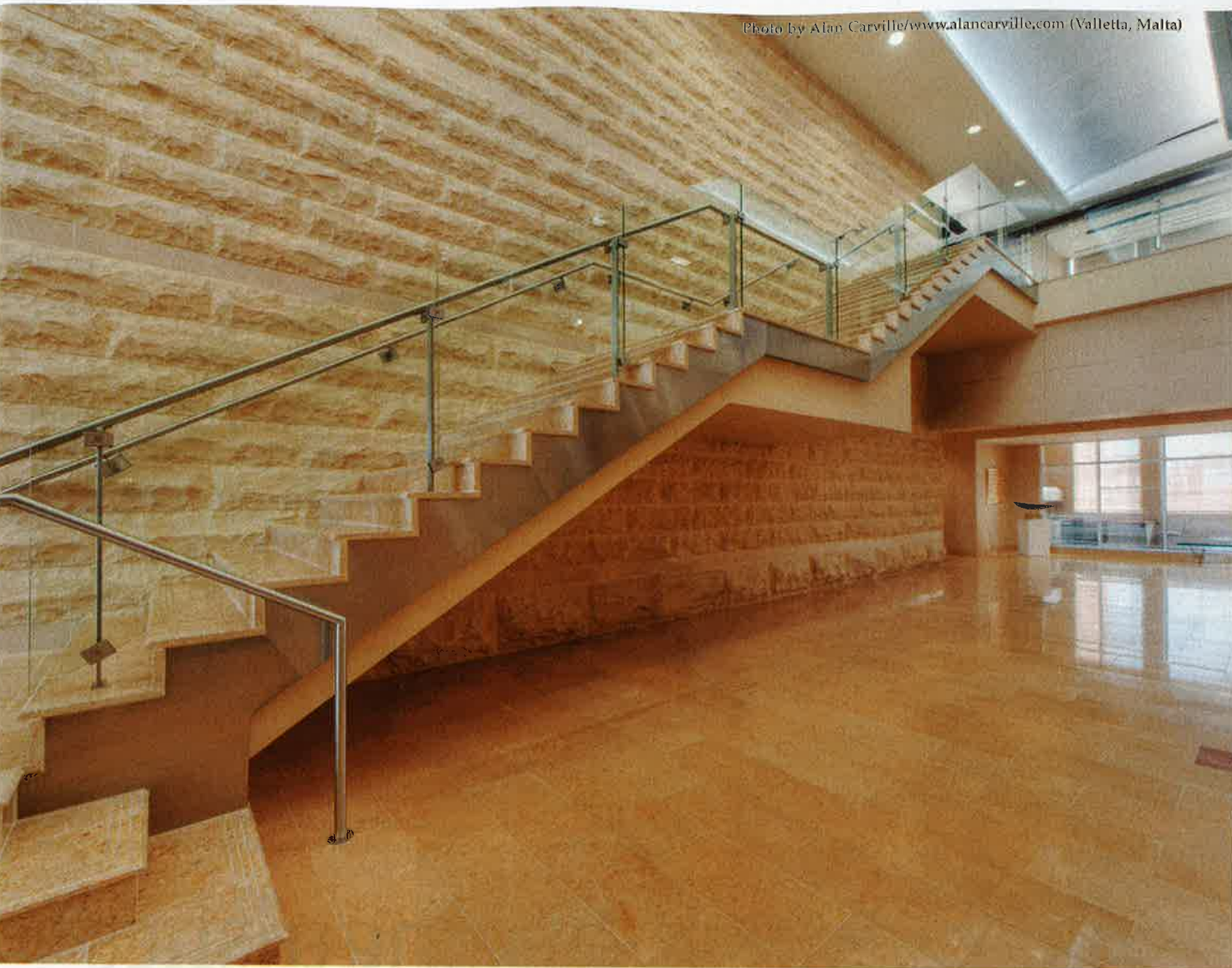
The wall behind the monumental stair features Frank Rockface limestone and honed Galala Classic limestone.
